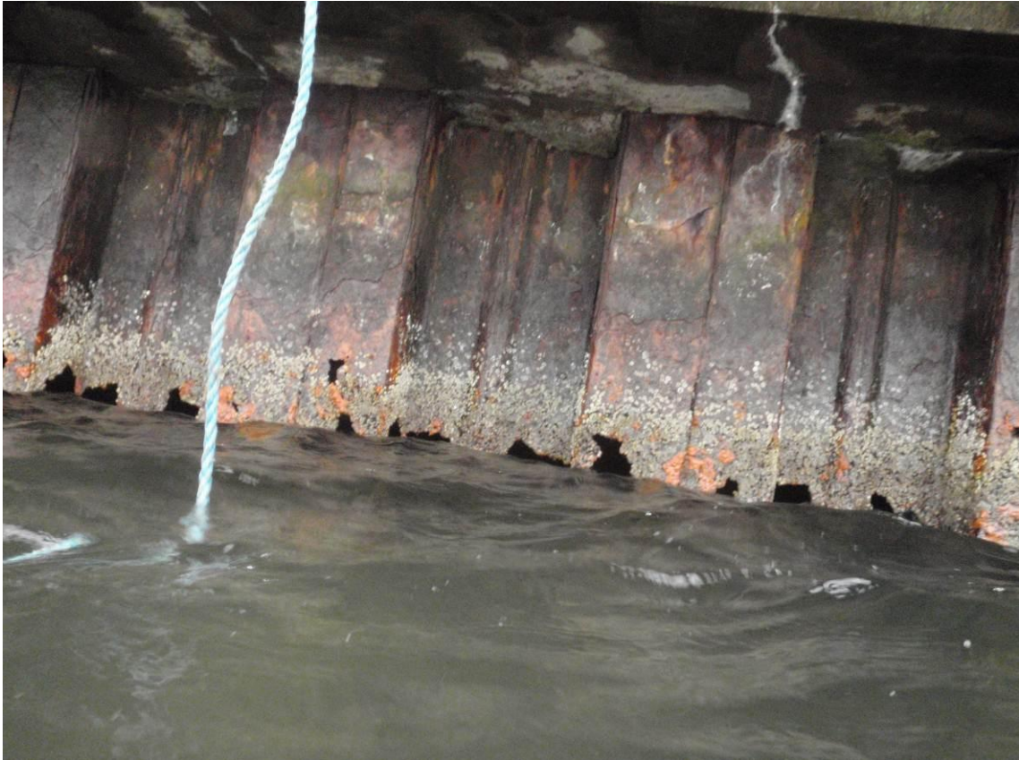
Figure 1: Sheet pile wall on the Swedish east coast suffering from severe corrosion (Joakim Brogstam, MarCon Teknik AB)
