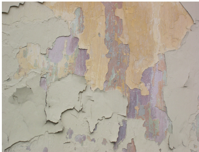
Figure 2. This detail of a plastered facade, from a farmers house in the coastal region of southern Sweden, shows many of the old layers of paint in many different colors.
