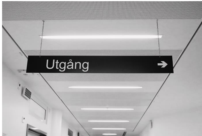
Figure 17. The exit sign with a pointing arrow at spot B.
