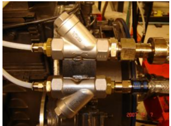
Figure 6 Pressurized air switching system built up by two check-valves
