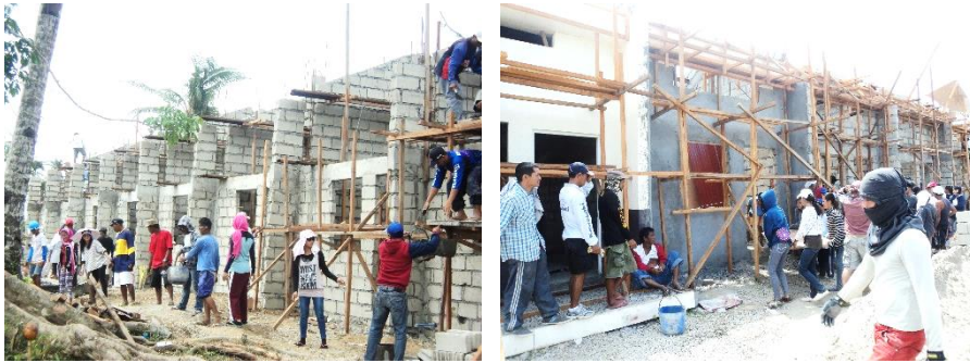
Figure 4.10 Users involved as unskilled labour, GK-Village in Barangay Pago, Tanauan. Pictures: by the author, March 10, 2014
