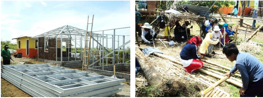
Figure 4.12 Housing solution and women working with bamboo, We Effect's pilot project in Barangay Dolores, Ormoc. The images show the construction method and women cutting, preserving and preparing bamboo for the walls. Pictures: by the author, March 6, 2014
