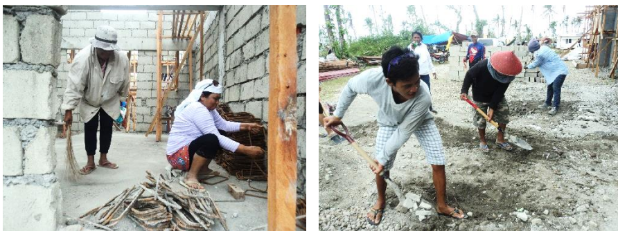
Figure 4.11 Users cleaning, reusing steel bars and preparing concrete, GK-Village in Barangay Pago, Tanauan. Pictures: by the author, March 10, 2014
