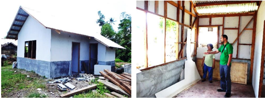
Figure 4.6 Community-driven reconstruction on-site in rural areas by the Relief and Rehabilitation Unit of the Archdiocese of Palo in Mayorga. Pictures: by the author, March 10, 2015
