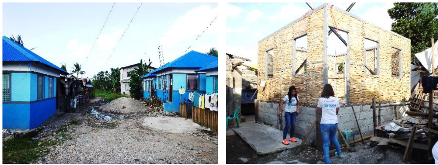
Figure 4.21 Agency-driven reconstruction on-site carried out by HFHP in Barangay Poblacion, Burauen. The housing typology and construction system of We Effect pilot housing were replicated. The owner decided to increase the height of the housing without receiving technical advice on housing adaptability for future expansion. Pictures: by the author, March 13/2015
