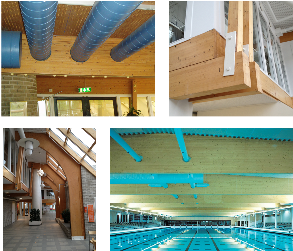
Figure 1.2: Ideon Science Park in Lund (top left, top right, bottom left) and indoor swimming pool in Västerås (bottom right, with permission from Martinssons Trä AB).
