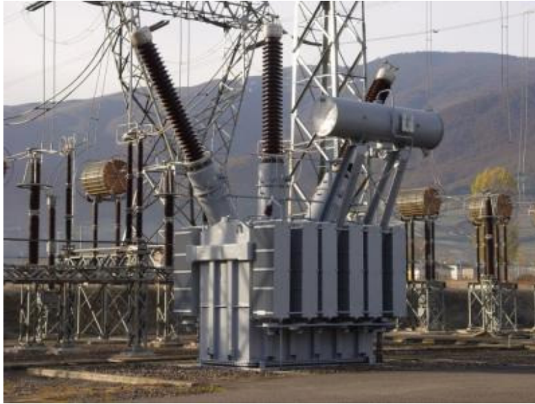
Figure 3. A power transformer in a 63/20 KV substation, West of Mazandaran
