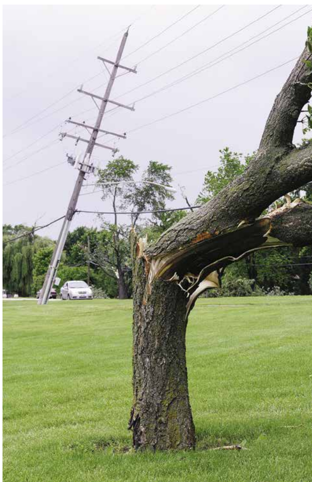
Figure 7. Damage to infrastructure caused by a wind storm (photo: Ken Schulze / shutterstock.com).
