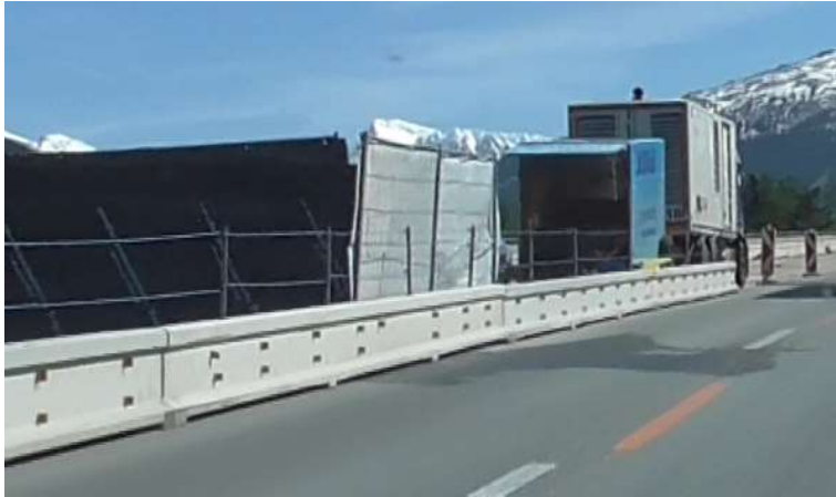
Figure 25: Small temporary vehicle restraint systems
