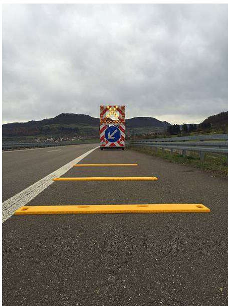
Figure 19: Portable rumble strips on hard shoulder
