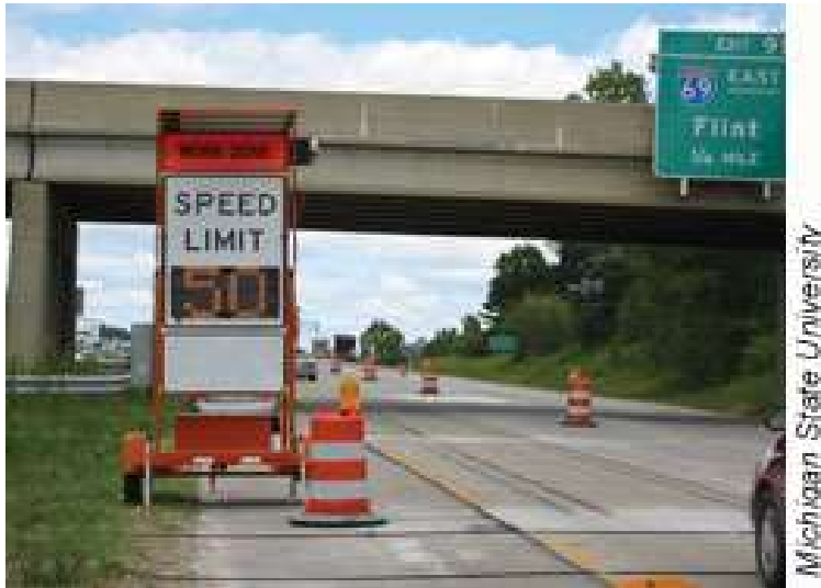
Figure 24: Variable speed limit sign in work zone
