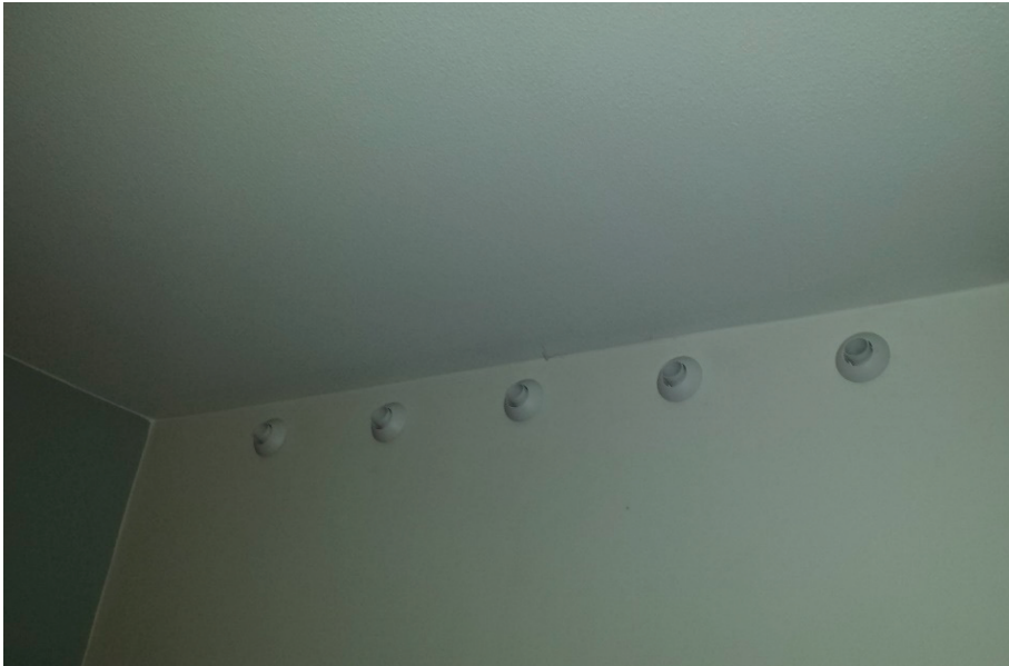
Figure A2.5: Pictures of covered supply and exhaust air devices inside apartments after installation.
