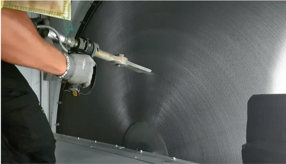
Figure A3.1: Cleaning process of heat exchangers – abrasive blasting with frozen CO 2 .
