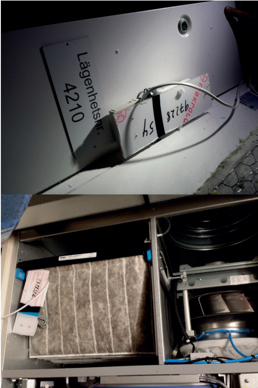
Figure A2.8: Pictures of sensor placement in ventilation system after renovation.
