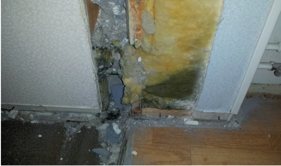
Figure A1.3: Mold growth in internal insulation layer of an exterior masonry wall.
