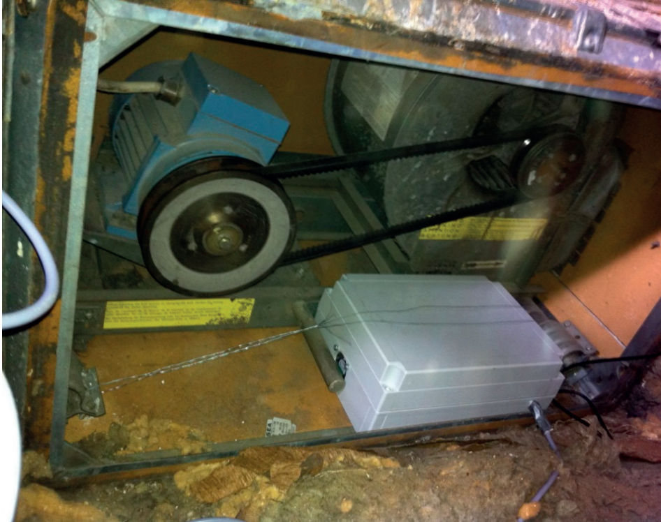
Figure A2.6: Picture of sensor placement in ventilation system before renovation.
