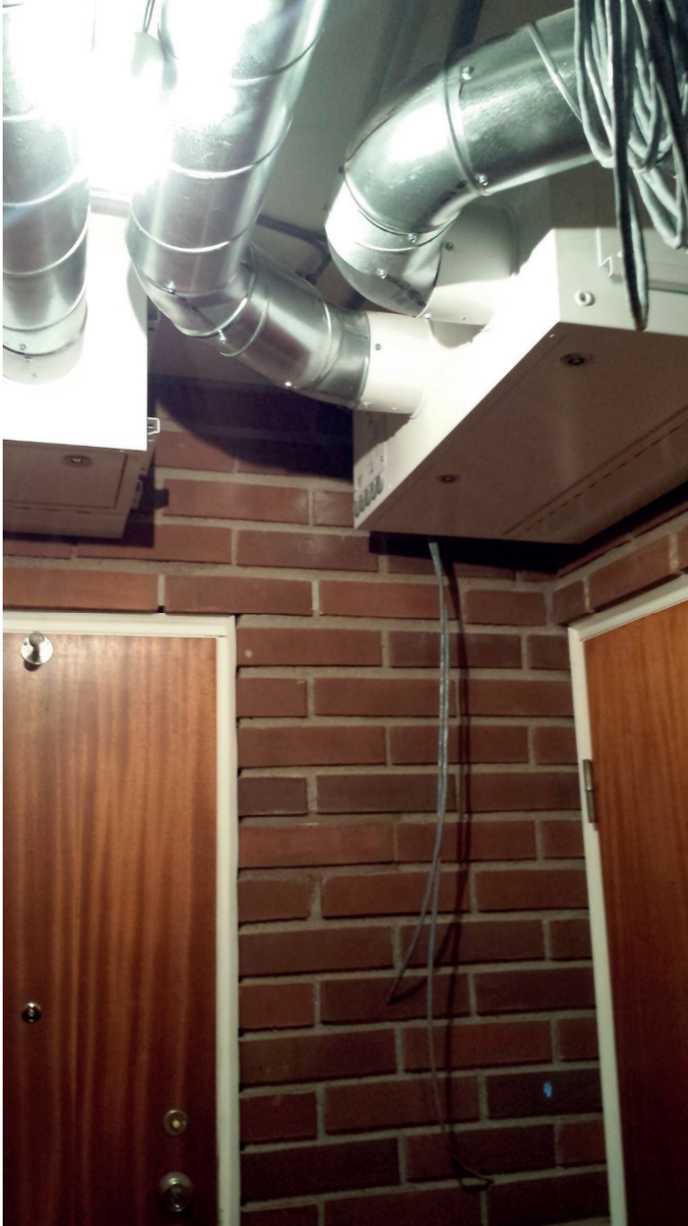
Figure A2.2: Picture of sensor and damper box in hallway during installation.
