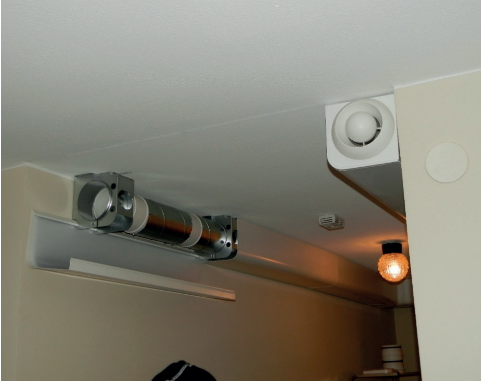
Figure A2.3: Picture of supply and exhaust air ducts in apartment during installation.
