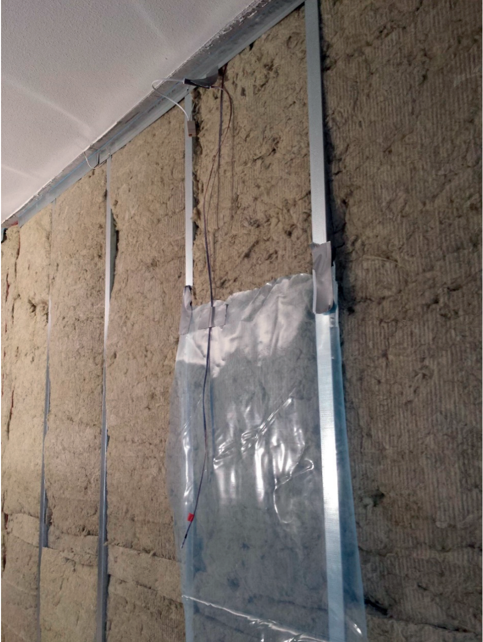
Figure A1.6: Sensor installation on both sides of vapor barrier applied with new internal insulation with steel studs.
