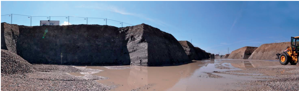
Figure 4.9: Photograph of the soil at the excavation site for the Linac tunnel [48].
