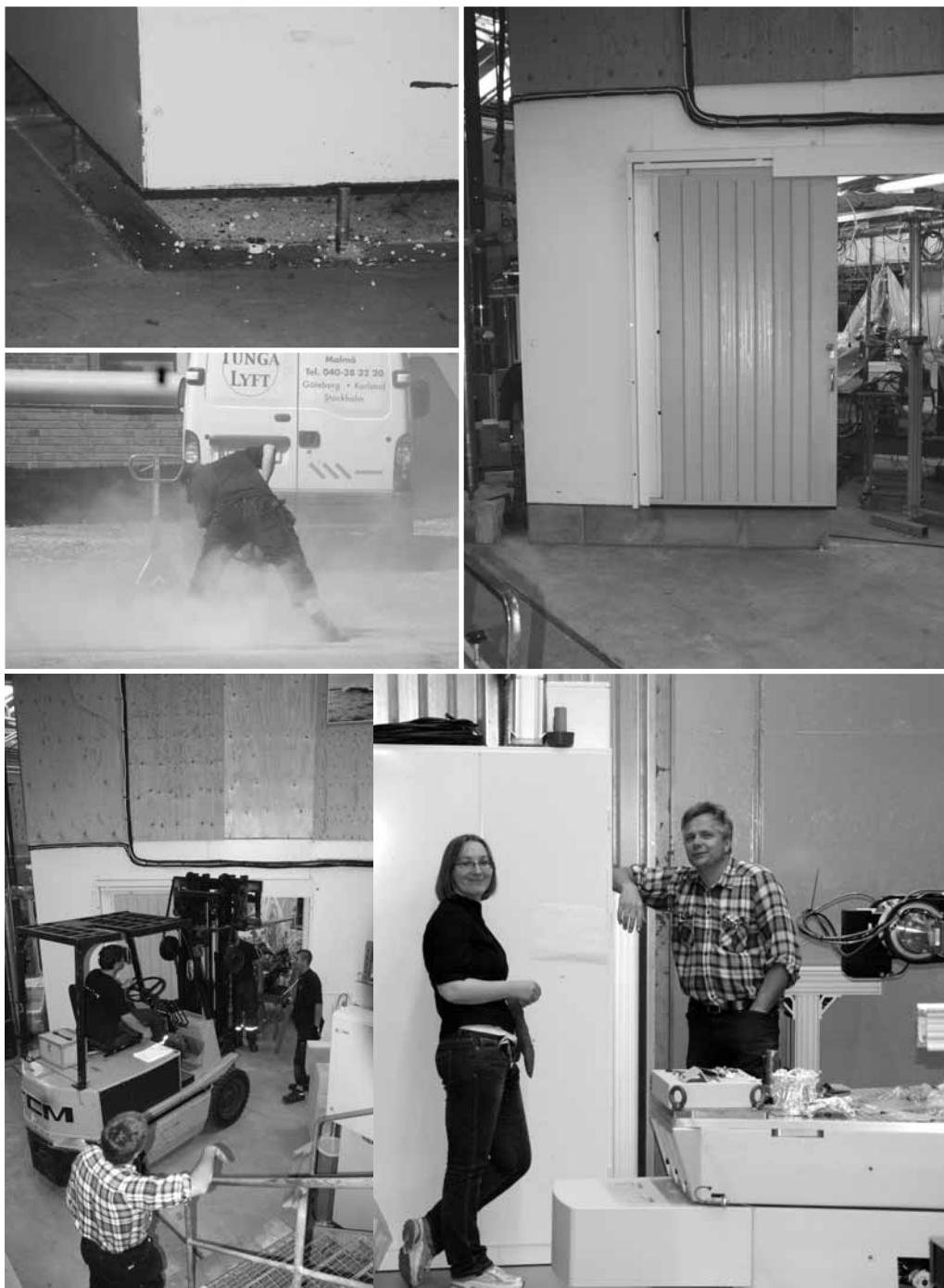
Redesign of the hutches around and at the beamline I711 itself. The present experimental hutch was raised 30cm and an additional office area was built on top of the redesigned beamline. Katarina Norén and Anders Månsson outside the hutch, 7 July 2010. Photos: Jeppe Christensen
