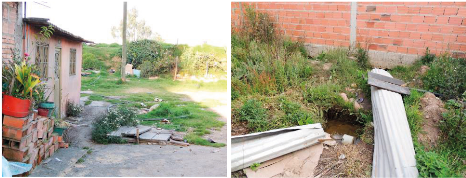
Figure 29. Wastewater disposal in San José I, Bosa
