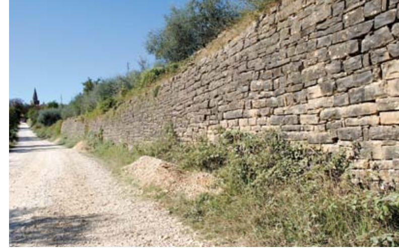
Figure 2: Dry stone retaining wall among a side road to Grožnjan (photo: Tanja Plešivčnik)
