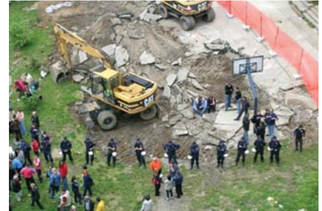
Figures 6: Residents are trying to stop construction workers from entering the park (source: www.petipark)
