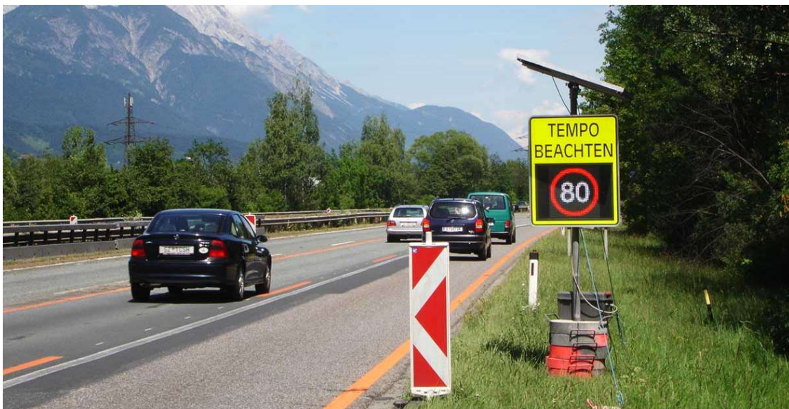
Figure 19. Variable speed limit sign at a work zone.
