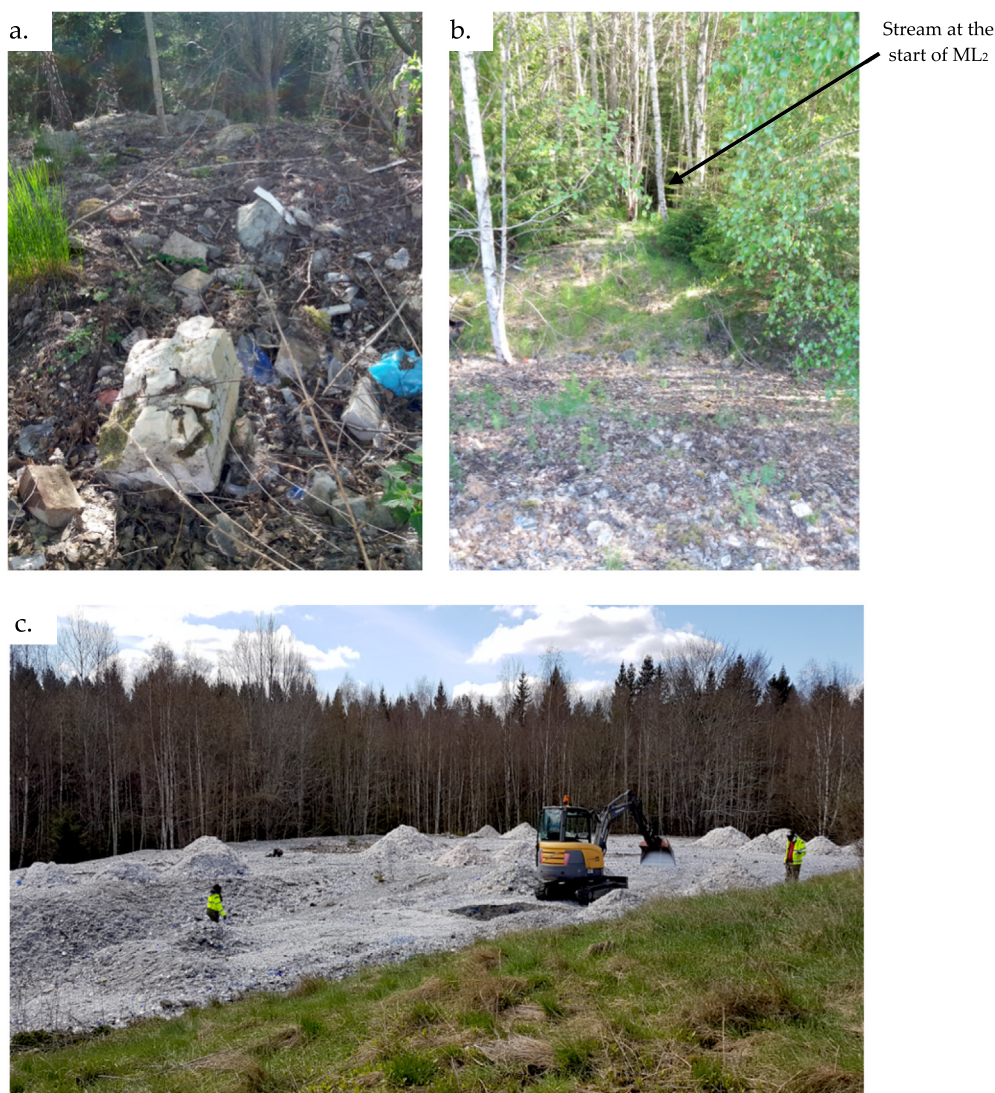
Fig. 4. Madesjö glass dump; (a) demolition waste heap at the start of ML 1 ; (b) start of ML 2 near the stream; (c) TP excavations across the dump.
