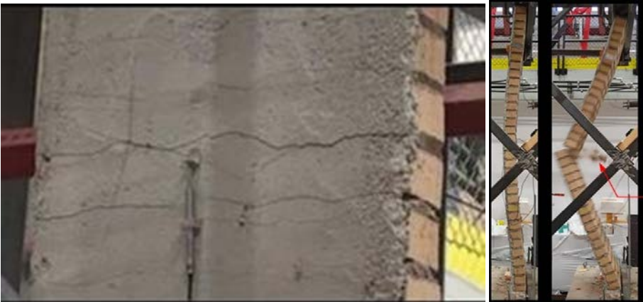
Figure B1_W5_3 Cracks at mid-height of the wall just before failure (left); Collapse of the wall (right).
