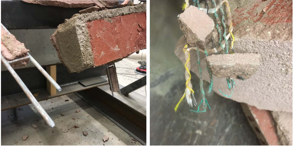
Figure 3.4 Tensile failure of strengthening, followed by collapse of the brick walls. Masonry reinforcement (left), high strength steel wire strip (right).
