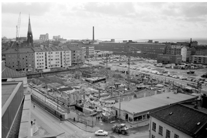
Figure 19. Opening up space for the Domus department store beside Södergatan In order to build the new department store, all the old buildings on the block were razed to the ground.
