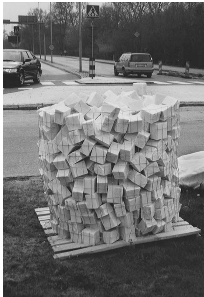
FIGURE 5. White marble paving stones ready to be laid at a pedestrian crossing in Lund. Photo by author.
