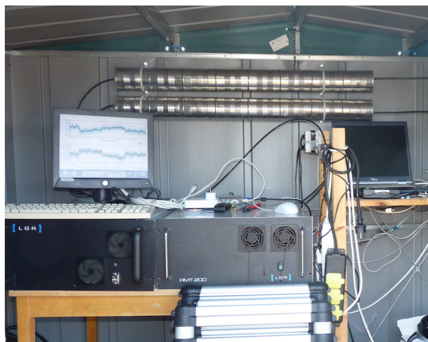
Figure 3: The inside of the small hut located close to the EC tower. Mixing volumes are visible in the top of the photo and the gas analyzer (LGR) in the bottom left corner.
