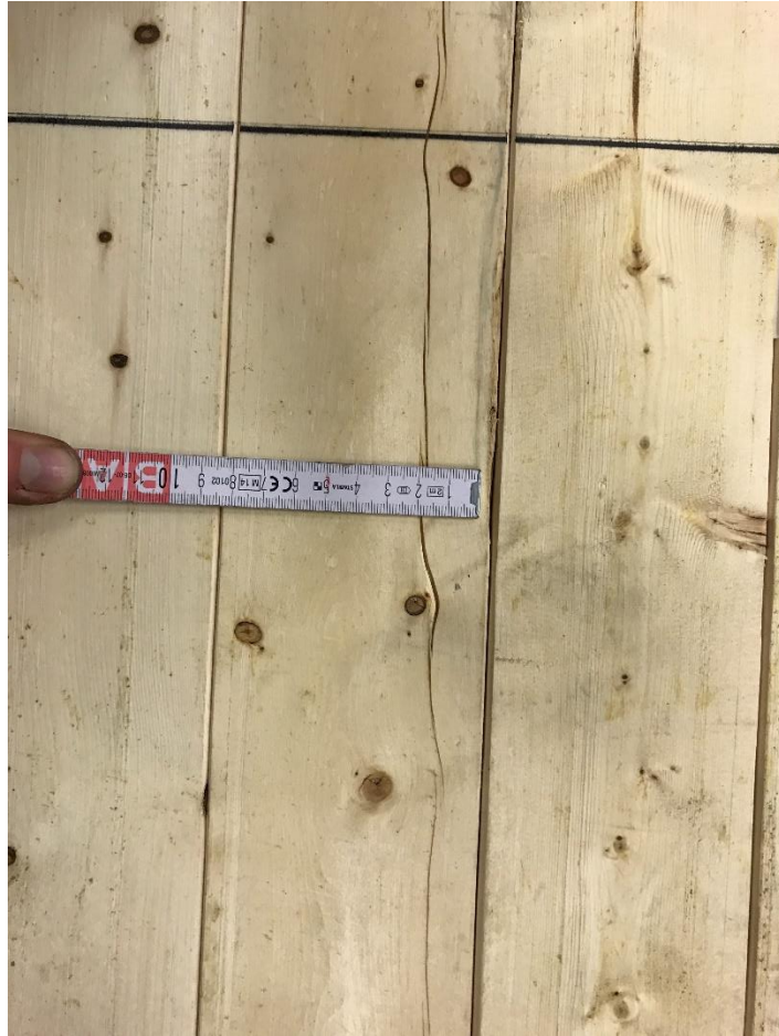
fig. G-3. A thin but long crack in the fire side of the MF-2 specimen.
