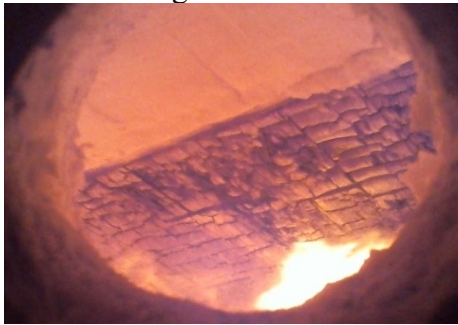
Initial stage of delamination
