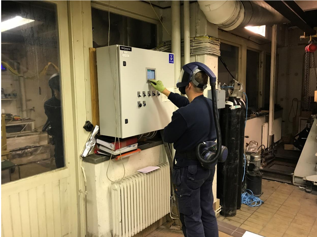
fig. G-23. Alar adjusting the burners inside the furnace from a control panel.
