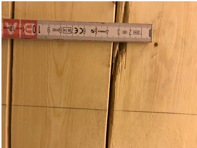
fig. G-4. A larger crack in between boards of the fire side of the PUR-B1 specimen.
