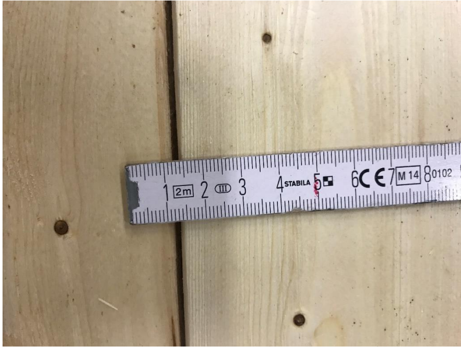
fig. G-5. Fire side of MF-1 specimen. For some specimen, the gaps between some boards of the surface lamellas was quite severe.
