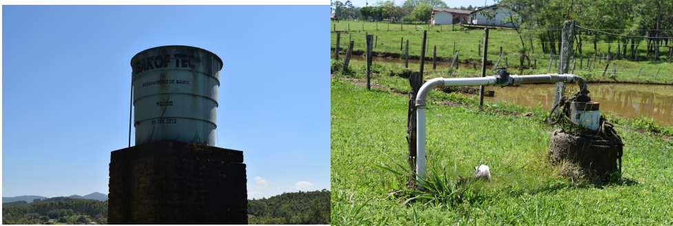
Figure 20 and Figure 21. Water reservoir and groundwater well of the Cabriúva system.
