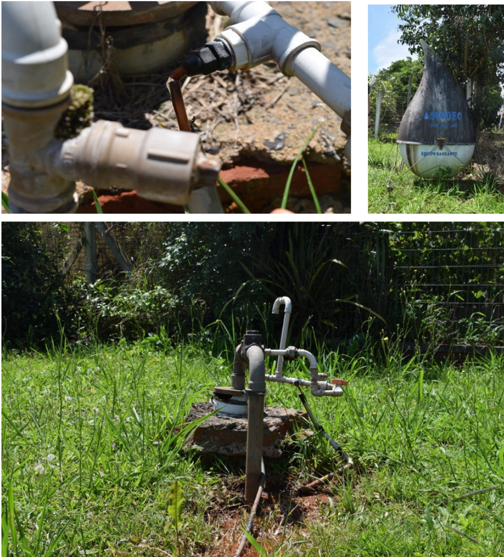
Figure 23, Figure 24 and Figure 25. Chlorination hose with damage, old chlorination tank and groundwater well of the Assodec Tristão system.
