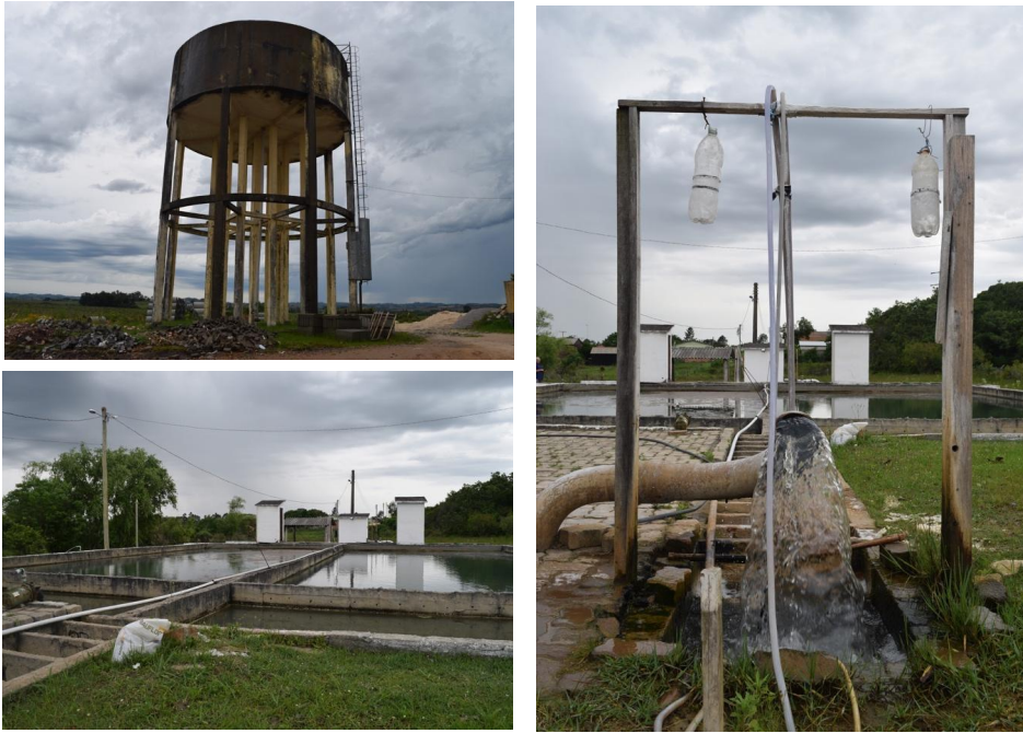
Figure 40, Figure 41 and Figure 42. Water reservoir and treatment plant of the SAA system.
