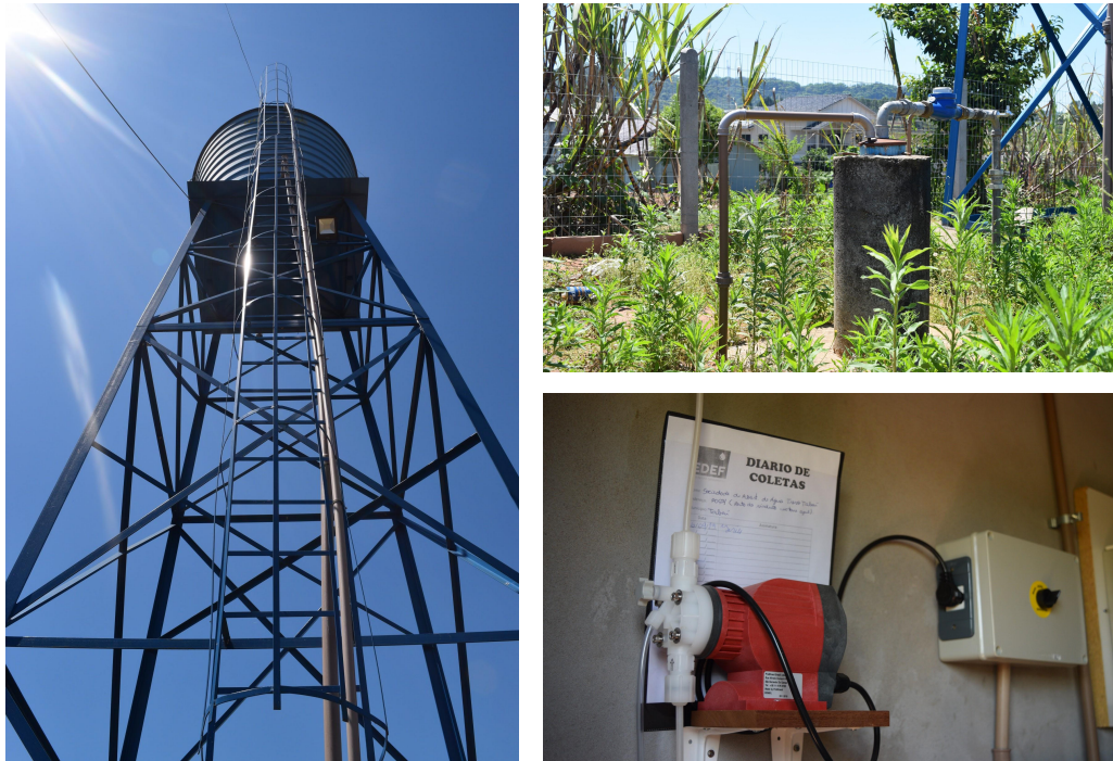
Figure 16, Figure 17 and Figure 18. Elevated water reservoir, groundwater well and chlorine disinfection system belonging to Sociedade Abastecedora de Água de Trevo Tabai.
