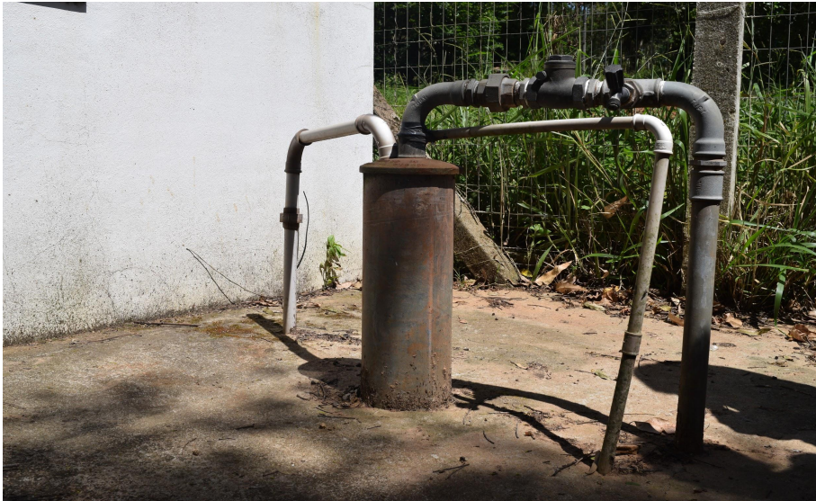
Figure 27. Groundwater well of Samambaia
