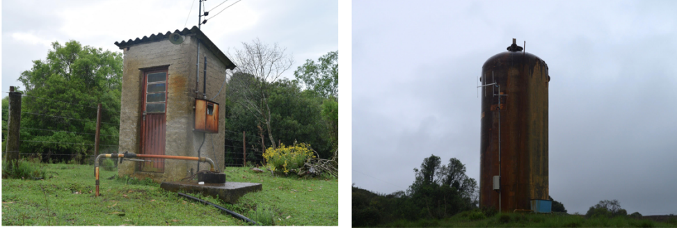
Figure 29 and Figure 30. Groundwater well and pumping house, and water reservoir in Laranjeiras.
