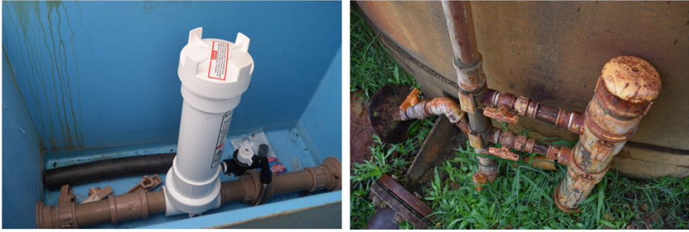
Figure 31 and Figure 32. New and old chlorination system by the water reservoir in Laranjeiras.
