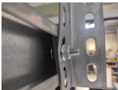
(a) Picture showing how the vertical support is connected to the C-beam
