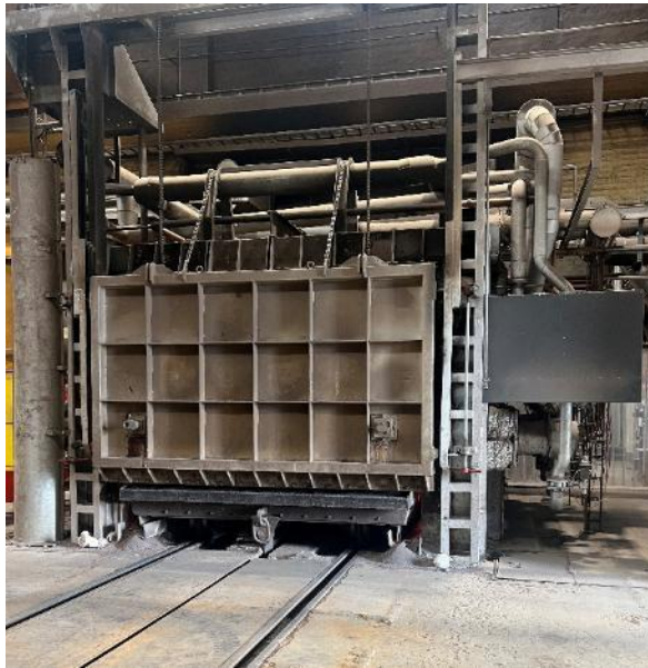
Figure 22: Car-type industrial furnace.
