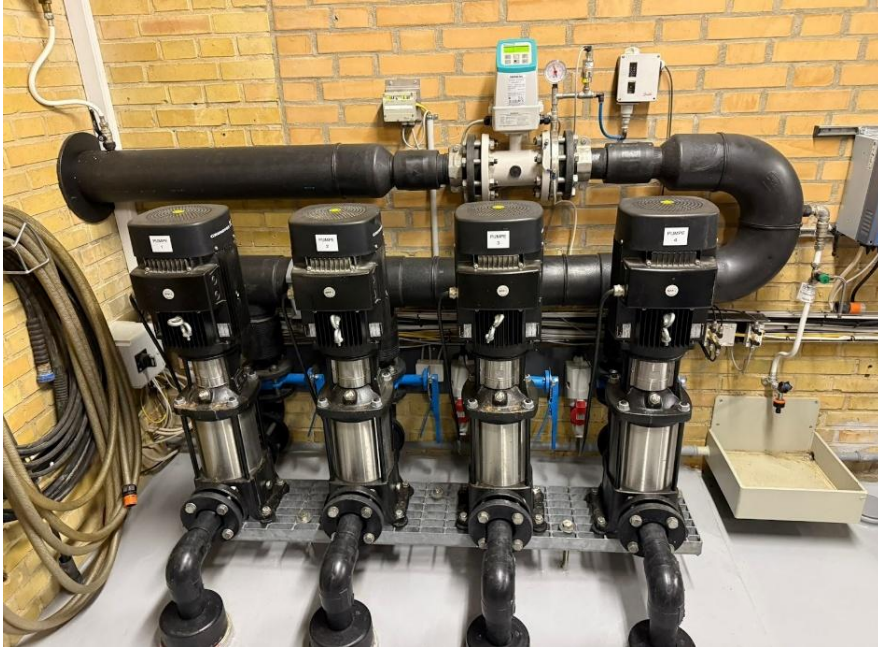
Figure 4.10. Four Parallel Pumps at the Waterworks
