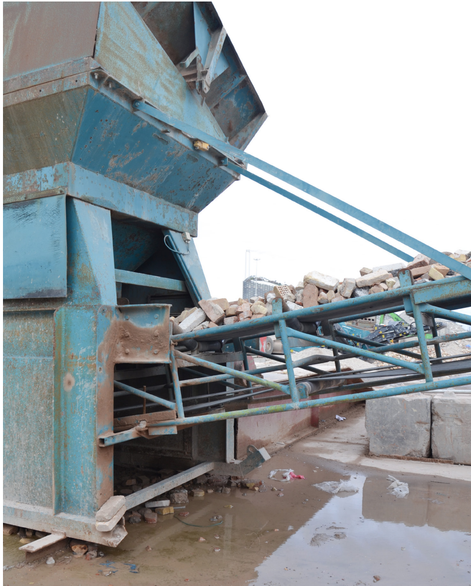
Conveyor belt transportation to sorting
