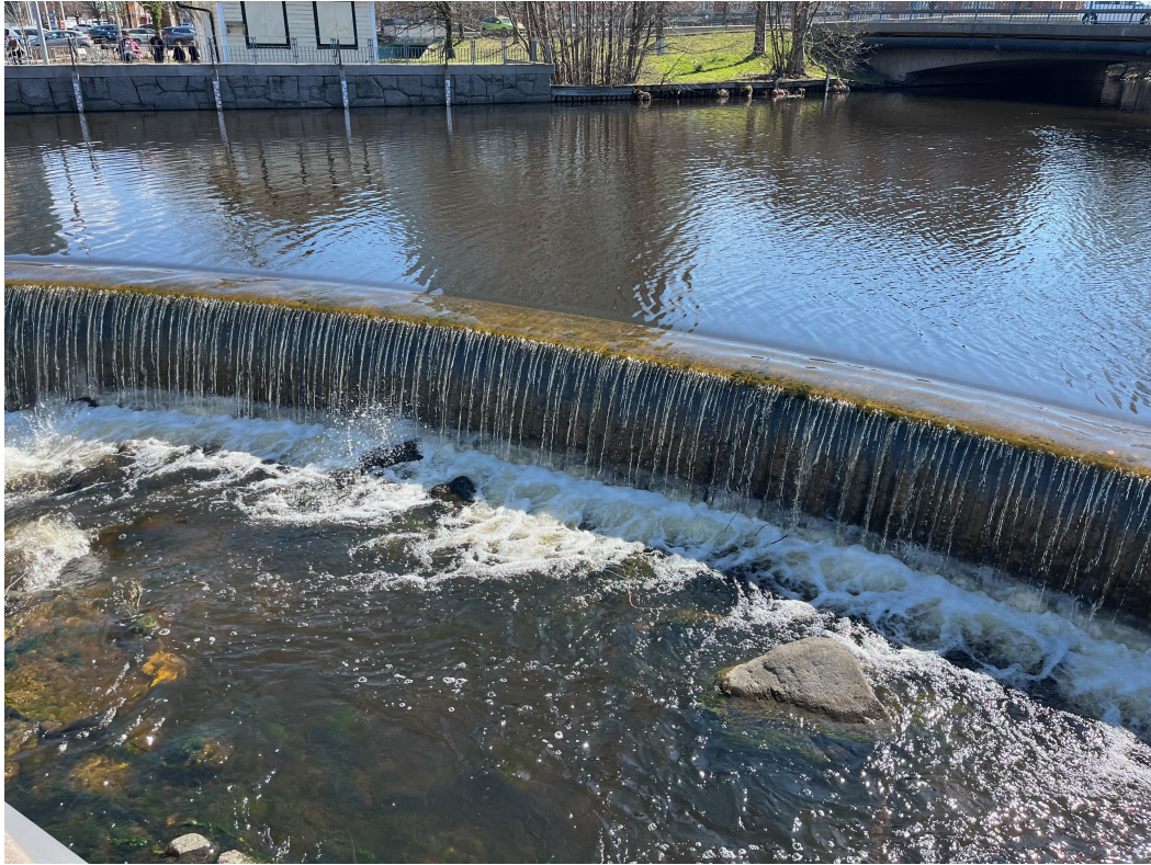
Figure 3.12: Picture of the weir along the fish passage at Gårda dämme. By Vera Åkerlund.
