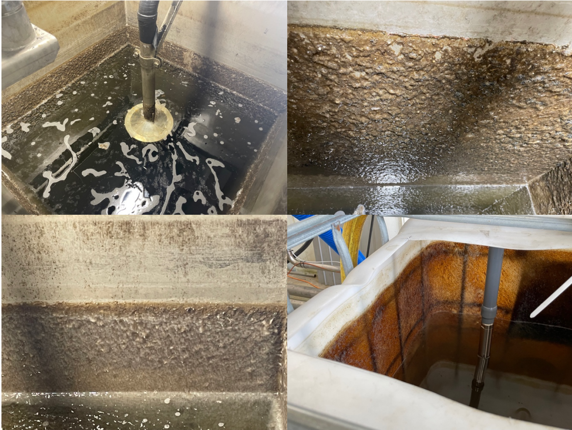
Figure 4.5. Pictures showing biofilm growth in the interior of the GAC filter and the influent IBC tank.
