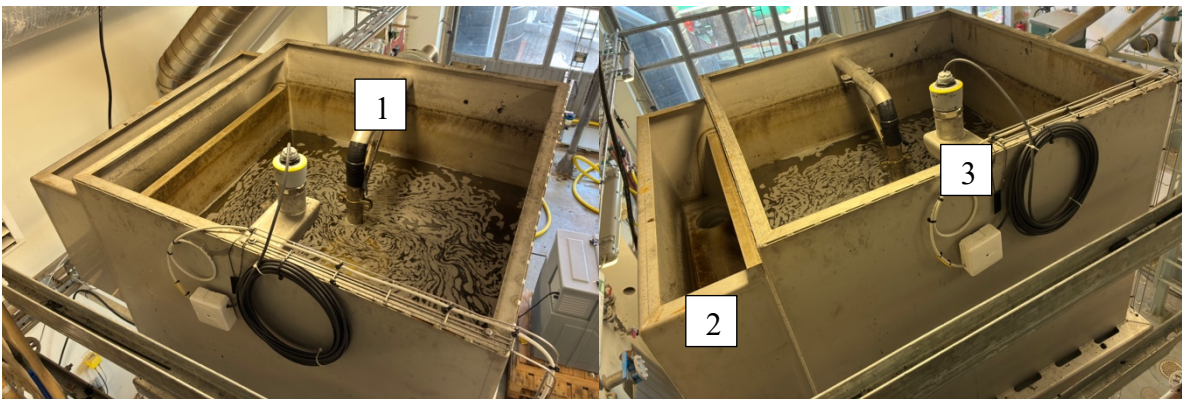
Figure 3.5. Pictures showing the top of the GAC. The numbers correspond to: 1 (influent pipe), 2 (overflow channel) and 3 (water level sensor).
