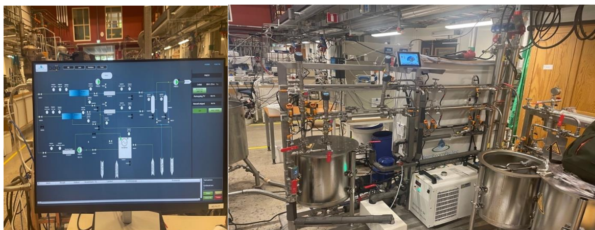
Figure 4.1. VMD configurations installed in tubular module with Human-Machine interface (HMI) screen (operator interface) for the pilot plant.
